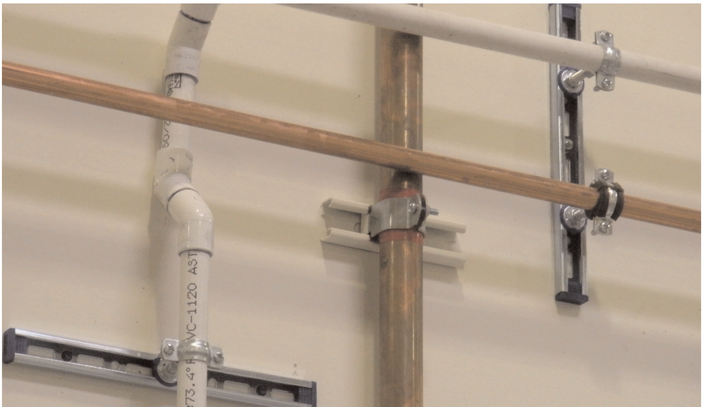
12" Euro Strut attached to wall with Sonic Cushion Clamps fixing PVC AND Copper Pipe.
