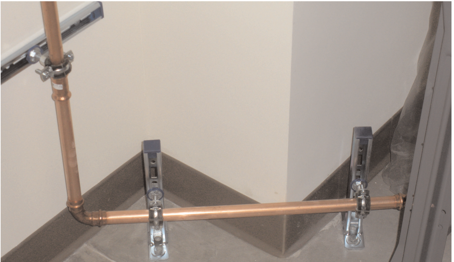
Euro Strut attached to wall with Sonic Clamps and Wall Hanger Brackets attached to floor with Sonic Clamps.
